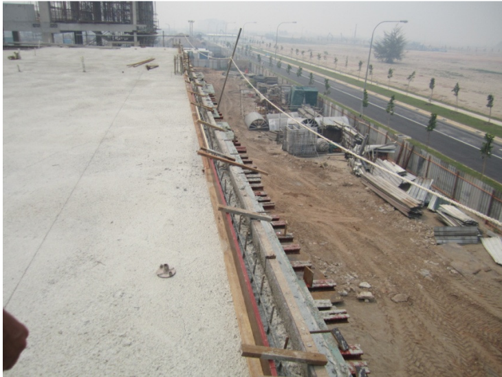
Unsecured openings without barricades
