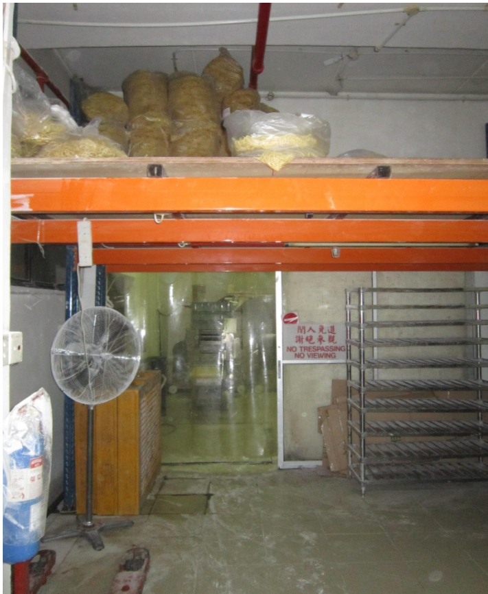
Open sides with a lack of barriers at the sides of mezzanine floors and staircases
