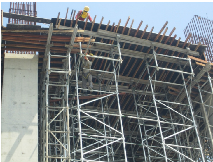
Lack of proper access to and from work areas
