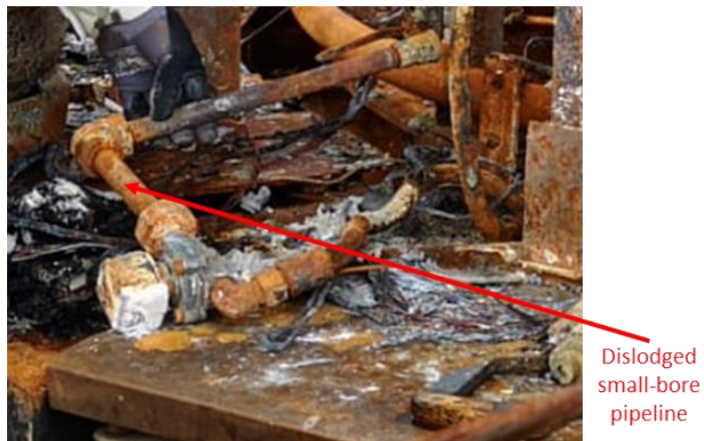
Figure 5. Close-up view of the dislodged ½” small-bore LPG pipeline
