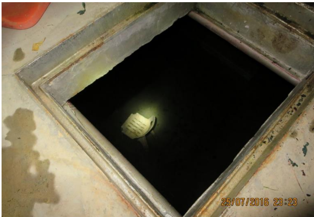
Photograph showing the view of the inside of the underground storage tank.
