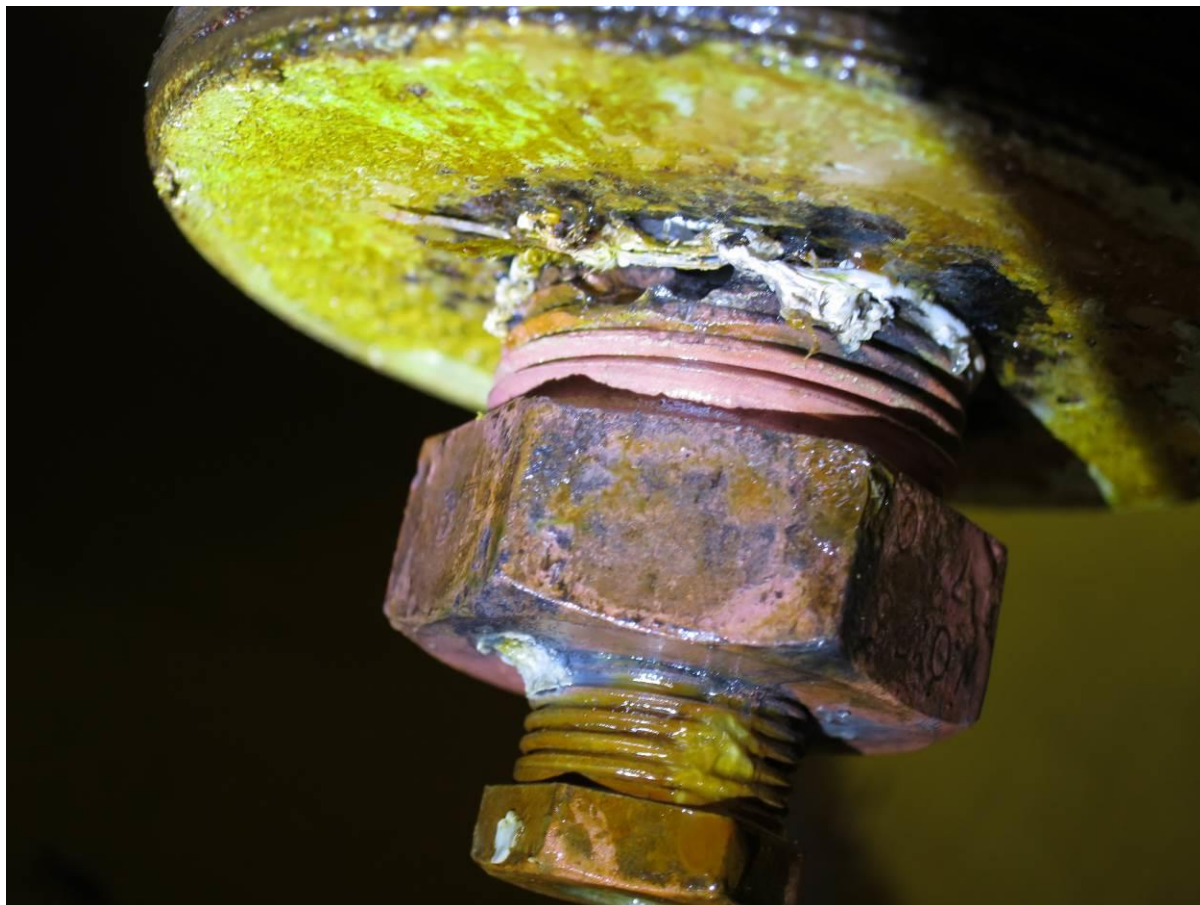
Photograph showing corroded fusible plug
