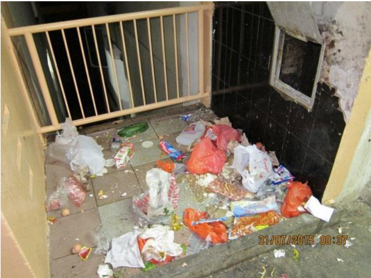
Photo C: Poor garbage disposals, leading to unsanitary living conditions.
