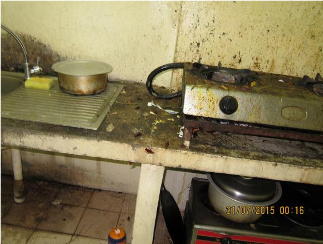
Photo E: Lack of hygiene maintenance at cooking area.
