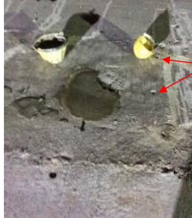
Examples of holes on the floor that the worker was to patch up with cement.
