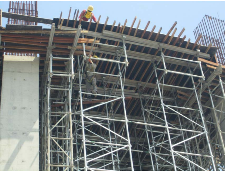
Lack of proper access to and from work areas
