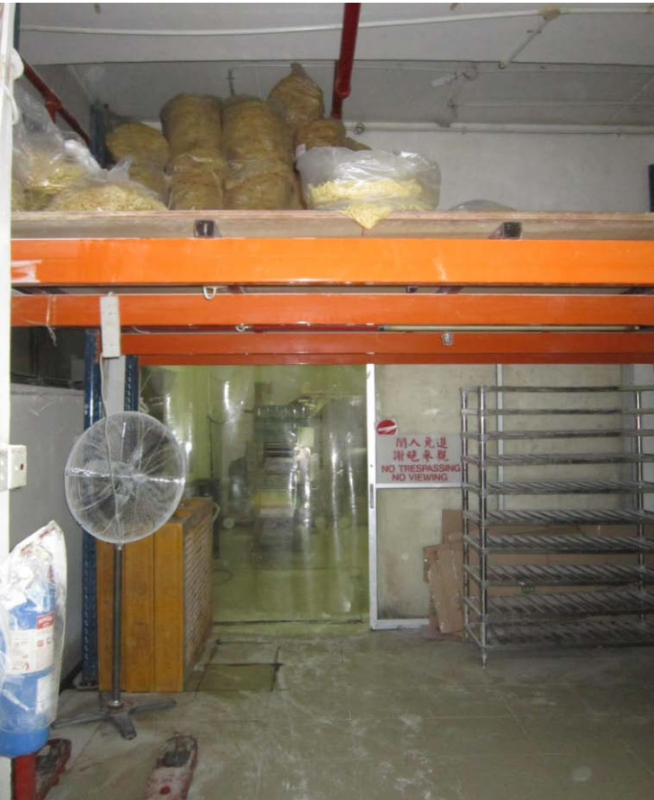
Open sides with a lack of barriers at the sides of mezzanine floors and staircases
