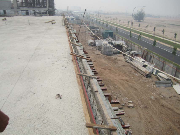
Unsecured openings without barricades
