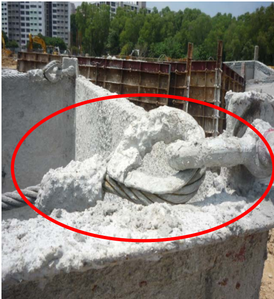
Figure 7a A poorly maintained lifting gear which could result in pre-matured failure of the lifting gear.
