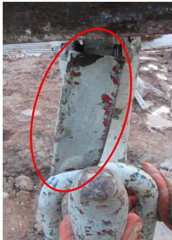
Figure 3 A defective safety hook latch of a crane (circled) which makes it ineffective in retaining of slings or other lifting devices.
