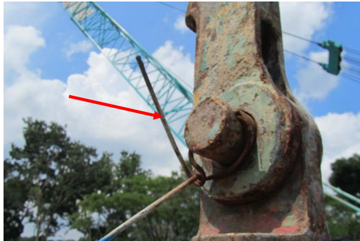
Figure 5 Improvised locking pin. Original locking pins, usually provided by the crane manufacturers, are purpose-built and designed to withstand the strains of lifting operations. Improvised equipment like this is prone to failure during lifting operations.
