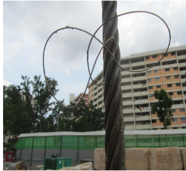
Figure 2b A deformed wire rope of a crane which may result in uneven stress distribution in the rope.
