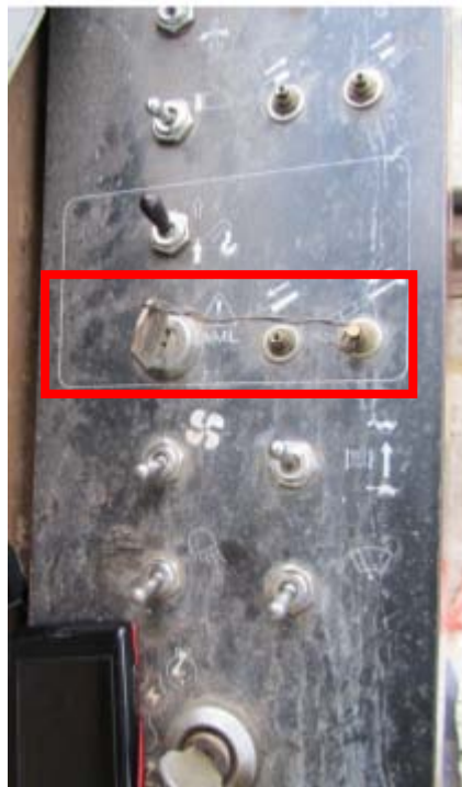
Figure 1. A malfunctioned control panel of a crawler crane. The crane operator of this crane would have to bypass safety features to operate the crane, thus increasing the risk of an accident.
