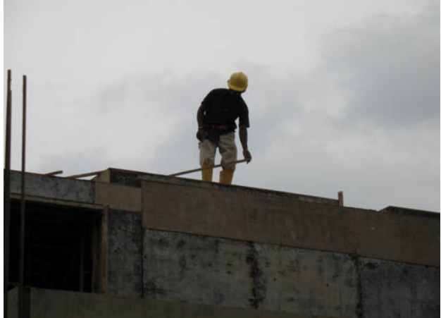
Worker installing guardrails at edge of building without any fall protection
