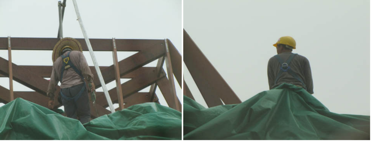
Harness worn by workers did not come with lanyards and snap-hooks for securing to anchorages
