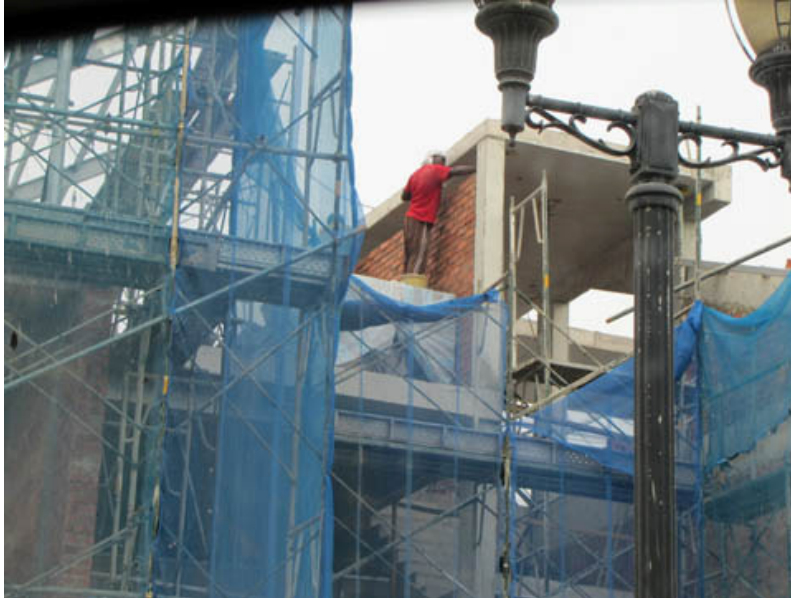
Fall protection not provided for worker
