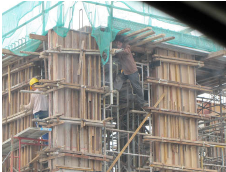
No proper work platforms for workers
