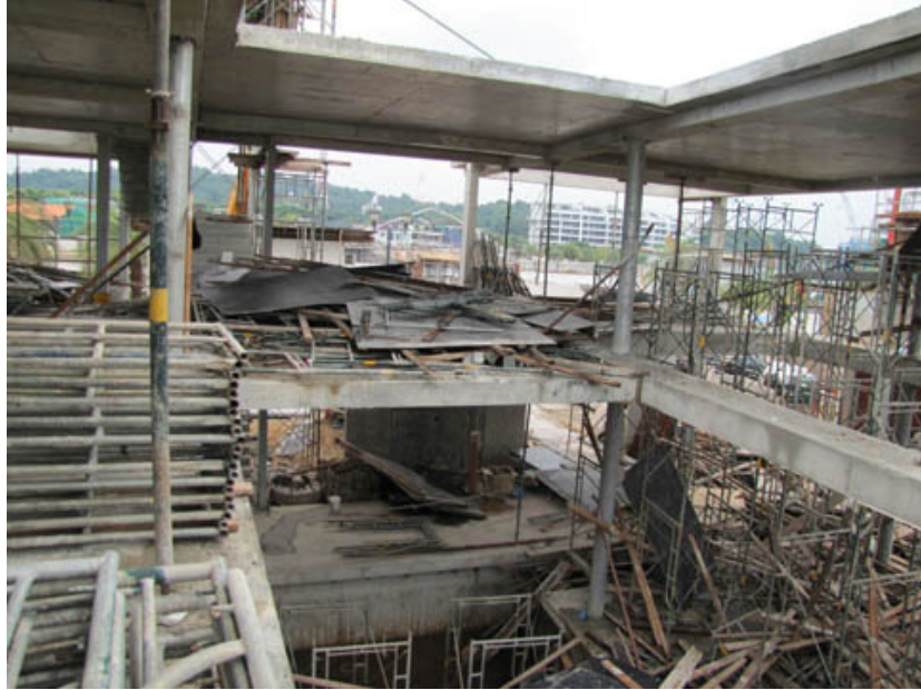
Edges of entire levels not barricaded to prevent persons from falling, as well as poor housekeeping with loose materials being placed close to the edges obstructing access
