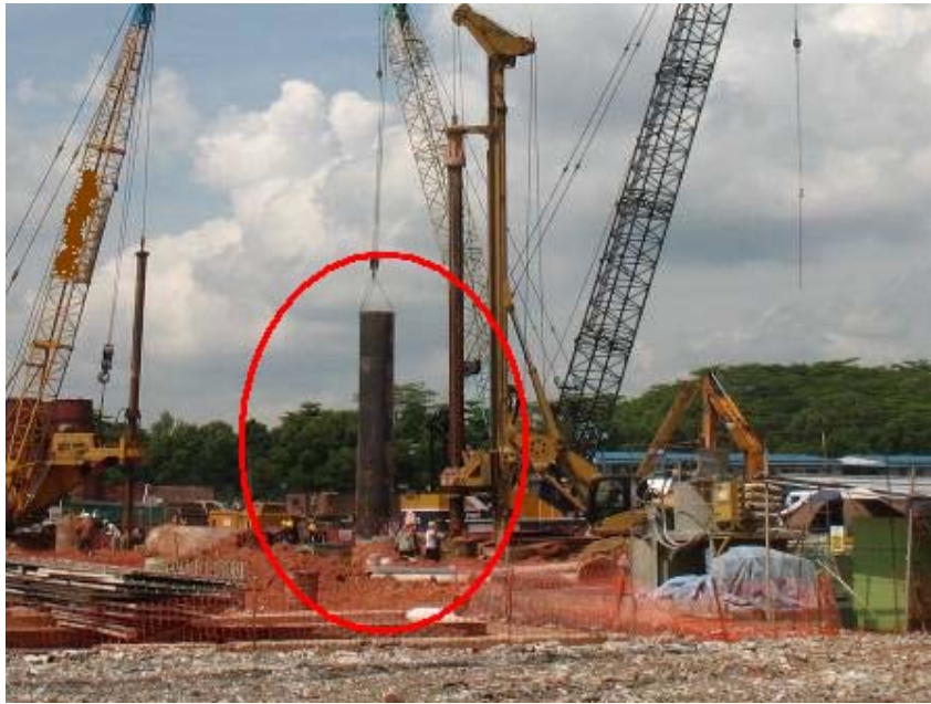
Figure 7: Improper use of crane
