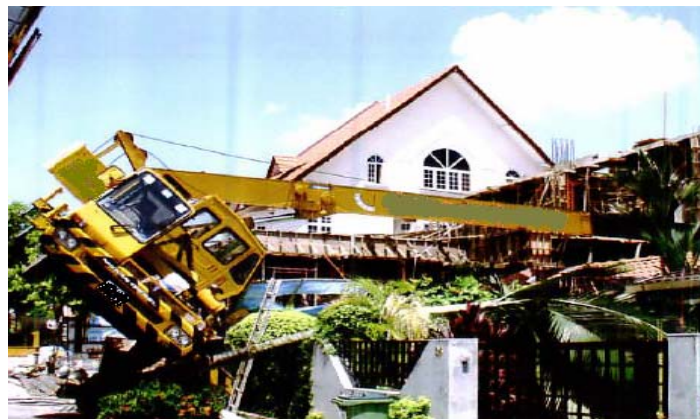
Figure 5: Collapse of crane due to overloading
