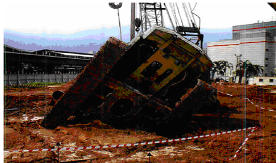
Figure 9: Collapse of crane due to soft ground condition
