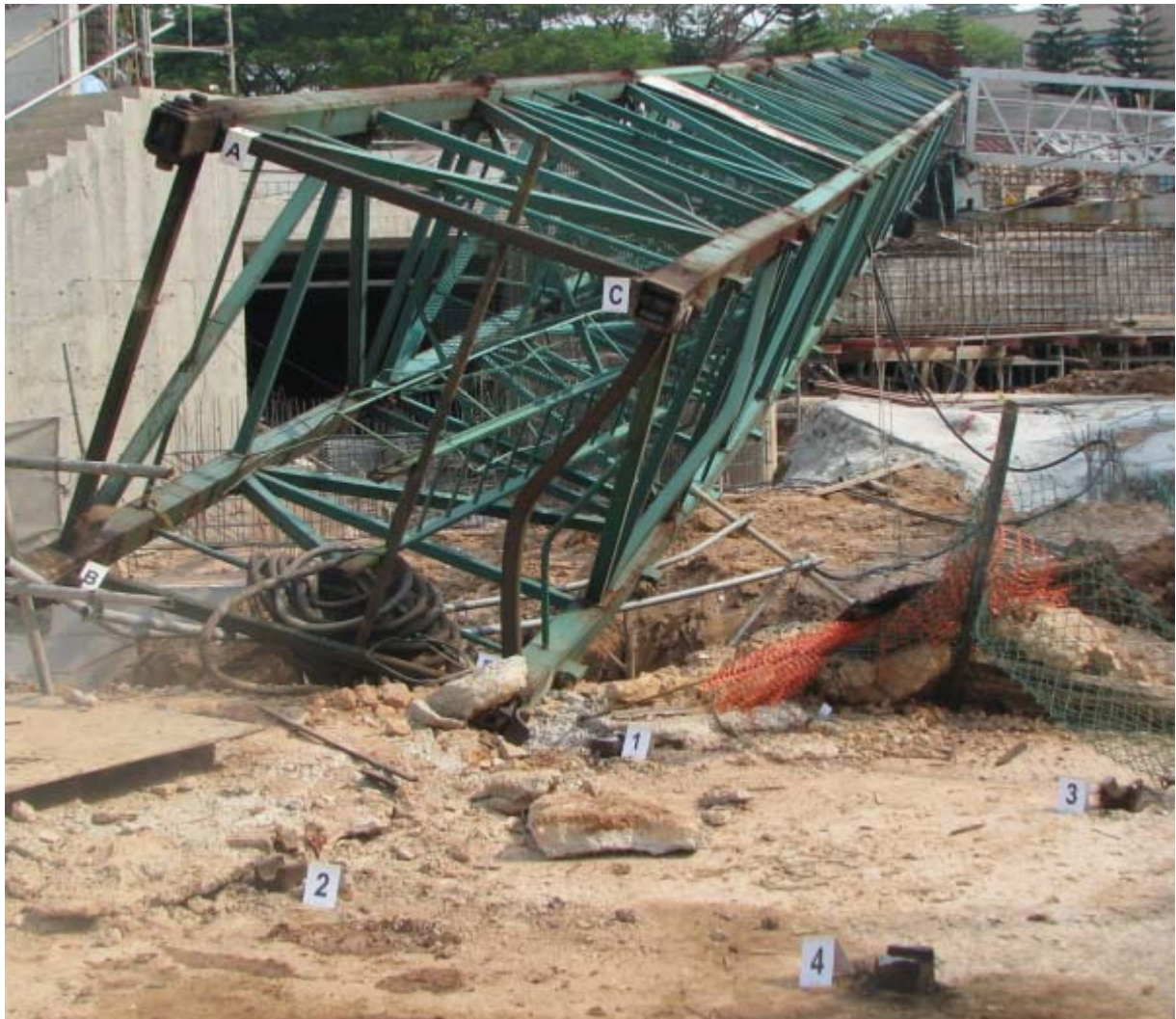
Photo of the collapsed tower crane and its base
