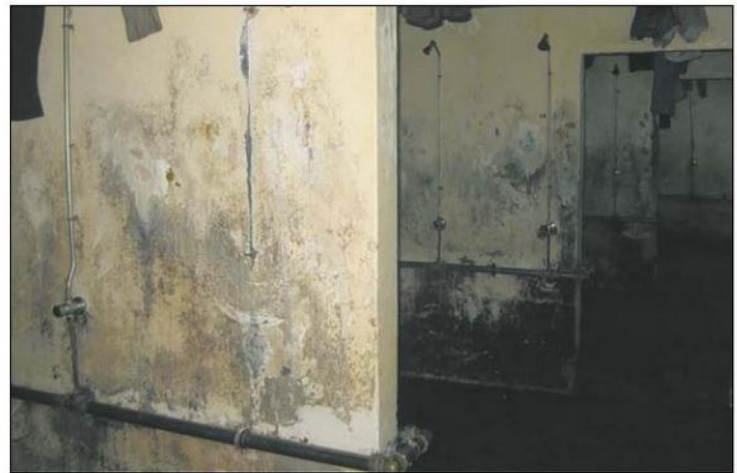
Shower facilities in a deplorable state in a foreign workers' dormitory. On Tuesday, five companies were found guilty of failing to provide acceptable accommodation for their foreign workers and other violations. PHOTO: MINISTRY OF MANPOWER
