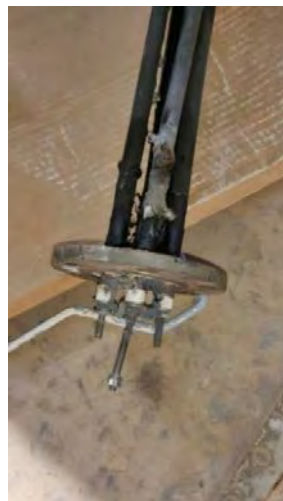
S-6: Photograph of damaged Heater No. 1, sent by Imam to Chua XD on 8 August 2020, 9:40am
