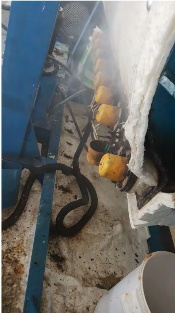
S-83: Photograph taken by Marimuthu on 24 February 2021 at 11:13am showing that the wiring of the damaged Heater No. 2 had been taped together with green tape, extracted from Marimuthu's mobile phone
