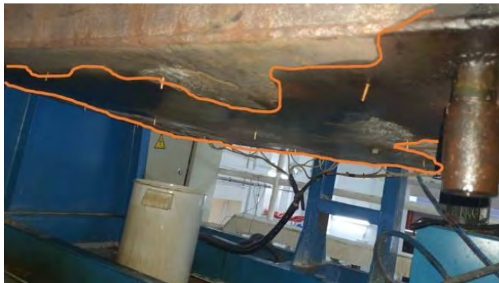
S-117: Photograph of the underside of the Mixer Machine near its front with the location of the oil stain that Murugan observed on 12 February 2021 outlined in orange colour
