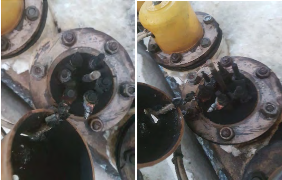
S-78 and S-79: Photographs of the burnt wiring connections of the damaged heater, sent by Marimuthu to Moe on 24 February 2021 at 9:04am via WhatsApp
