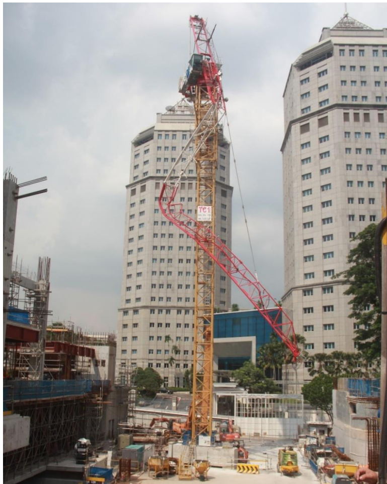
Figure 1 – General view of the TC after the accident
